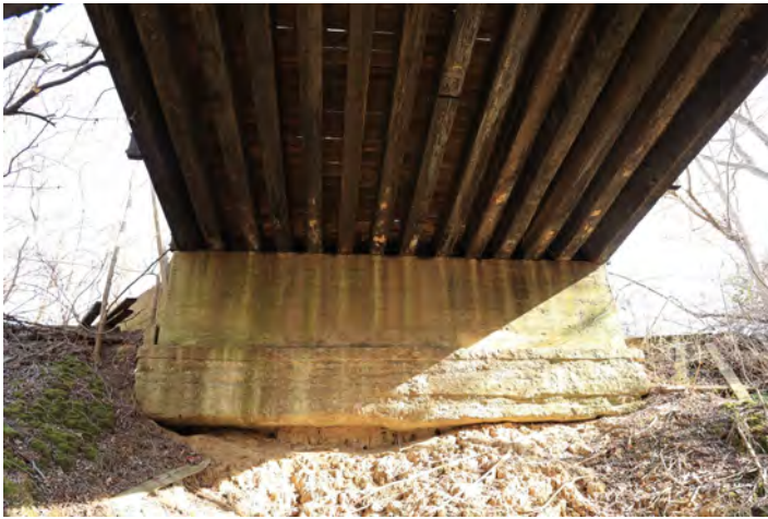
The eastern abutment undercut by erosion
