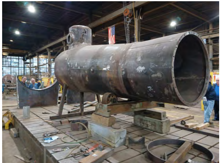
Another view of replacement F&J boiler, #112
