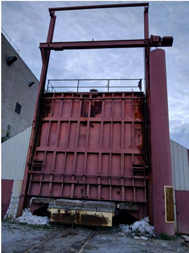
Front view, gas fired heat treatment oven
