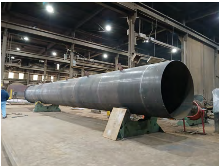
2nd section of flare stack
