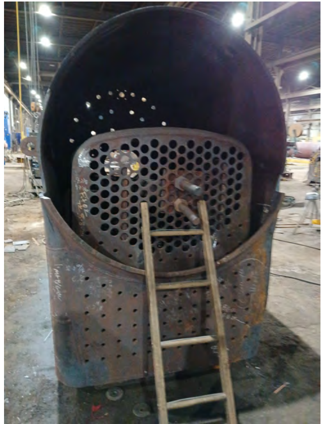
View looking inside fire box for replacement
